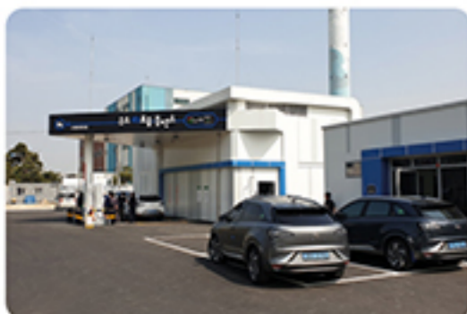
Ansan Charging Station
