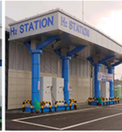
Seosan Charging Station
