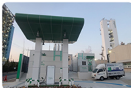
Ulsan APK Charging Station
