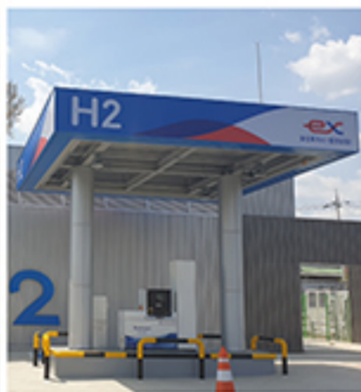
Eumseong Service Area Charging Station
